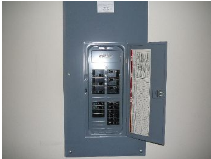
All of the circuit breakers appeared serviceable.
