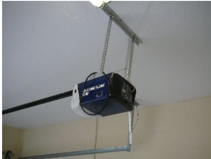
Chain drive opener noted.
