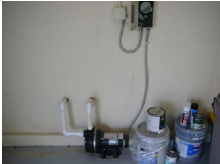
The sprinkler system operates with a control panel located in the garage.
