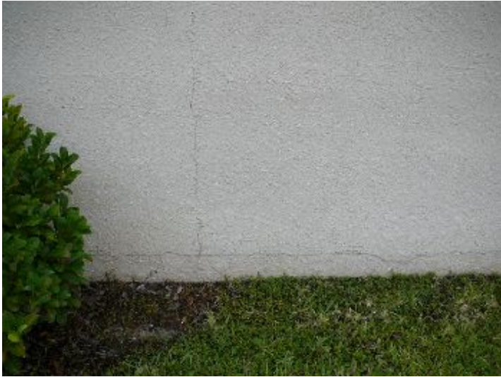
Cracks noted on the west exterior. Recommend consultation with qualified contractor to evaluate the condition of the foundation.
