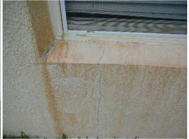
Cracks noted on the west exterior. Recommend consultation with qualified contractor to evaluate the condition of the foundation.
