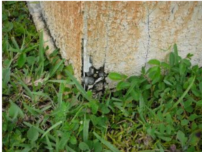
Common cracks observed, these may leak at any time.
