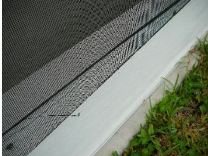
Screen loose on east side of porch.
