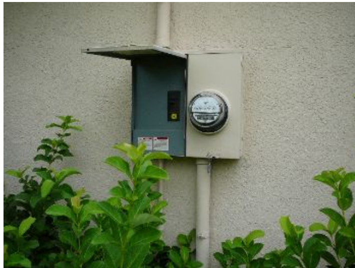
There is an underground service lateral noted.
